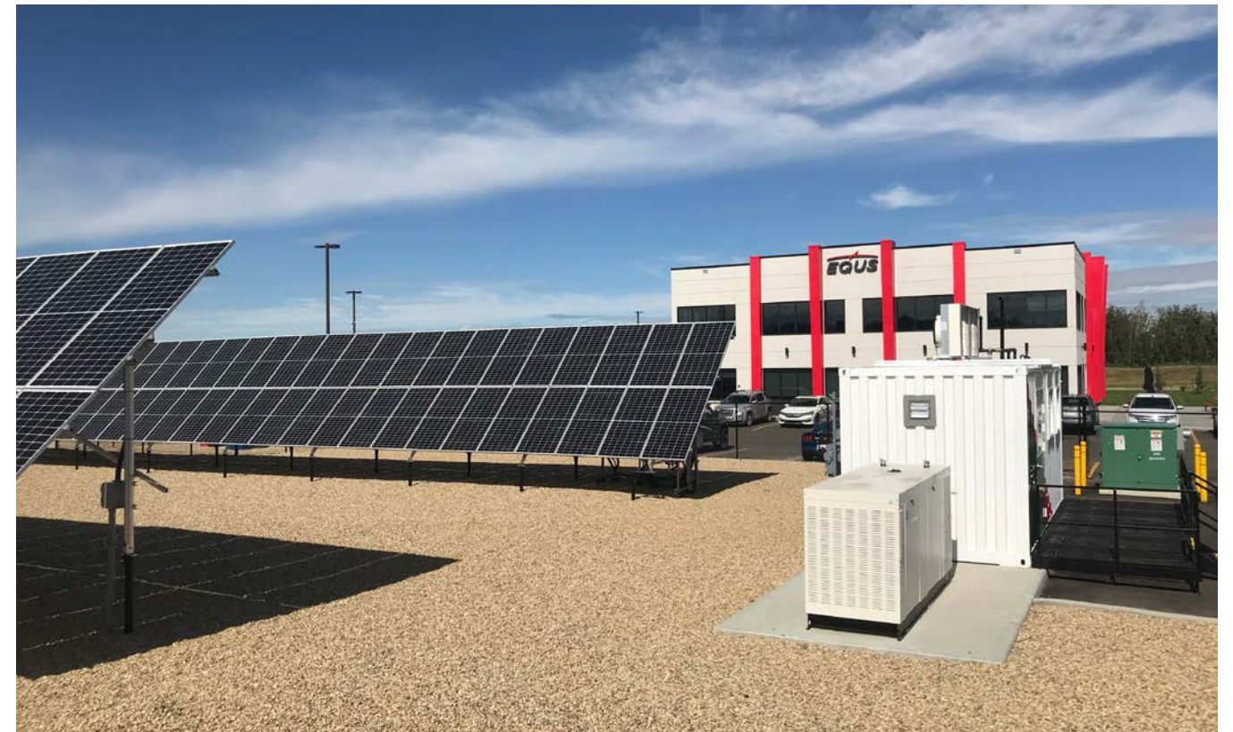
Our customer EQUUS, Alberta's largest cooperative power utility, uses a variety of energy efficient technologies to reach 'near net-zero' emissions performance at their head office.
