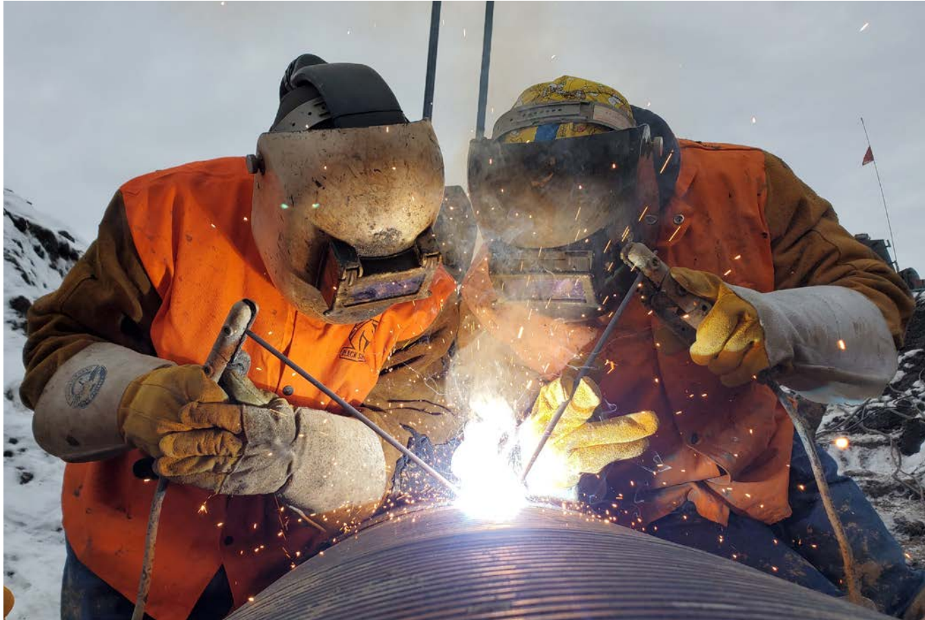
Construction of the Pembina-Keeyik Transmission Line was followed by long-term plans for inspection and maintenance, including mentorship and training opportunities for Indigenous communities.
